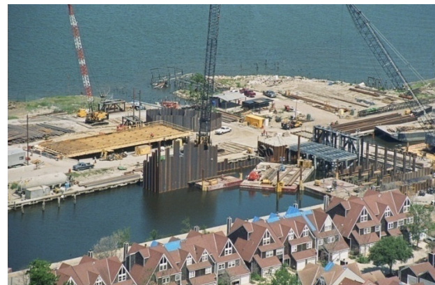
Sheet piles driven around perimeter of foundation. The sheet pile functioned as a cutoff wall and as a cofferdam
